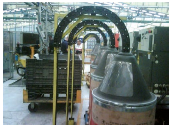
Application: Automotive production plant Drums at first floor above robotic installation
